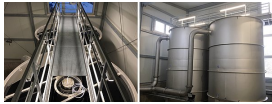
HUBER Active Carbon Filter CONTIFLOW® GAK as 4th treatment stage on STP Fridingen
