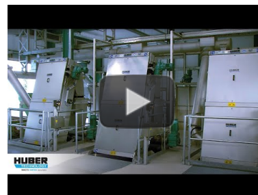
Video: Mechanical preliminary wastewater treatment - example: municipal WWTP Zwickau https://www.youtube.com/watch?v=SH3P8lpCDJM
