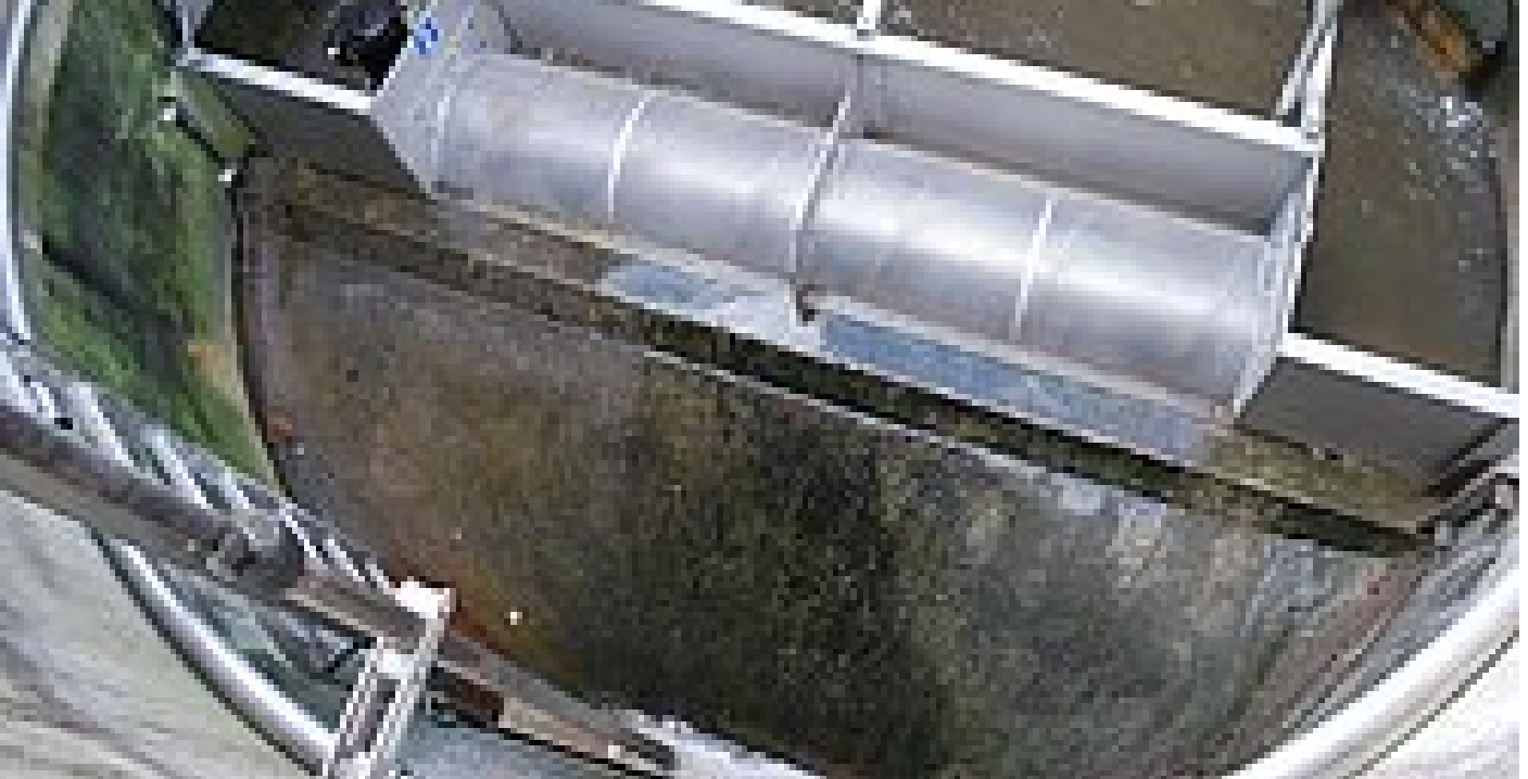
HUBER Storm Screen ROTAMAT® RoK2 in a stormwater overflow structure
