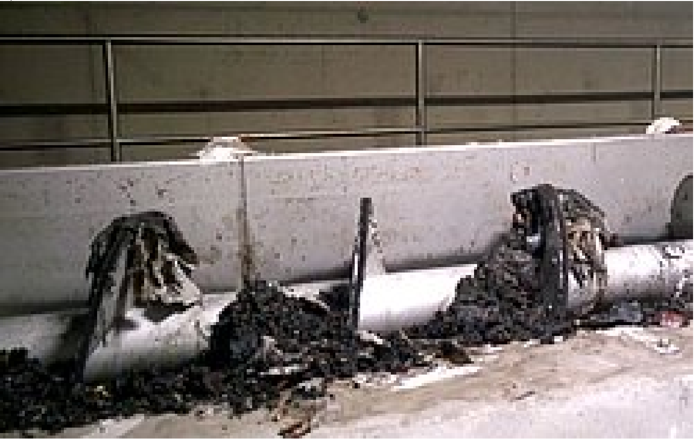
Increased screenings volumes on stormwater overflow discharge structures
