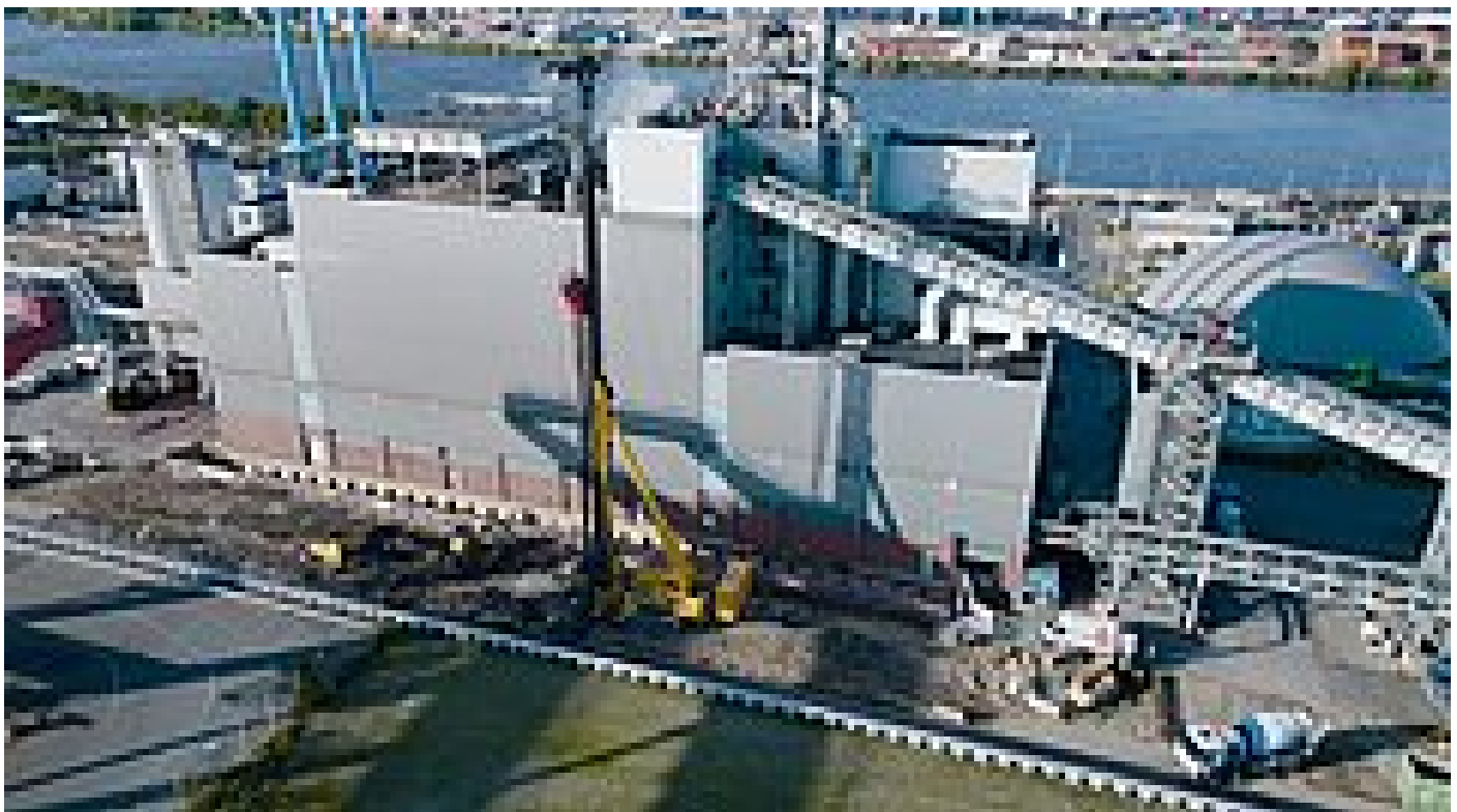
Aerial view of the construction work for the expansion of VERA II. (© HAMBURG WASSER)
