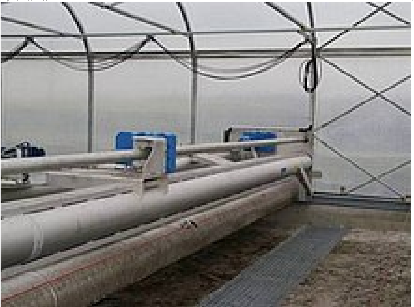
On its way back the sludge turner can drop the dry sludge into a screw that is installed below ground level.
