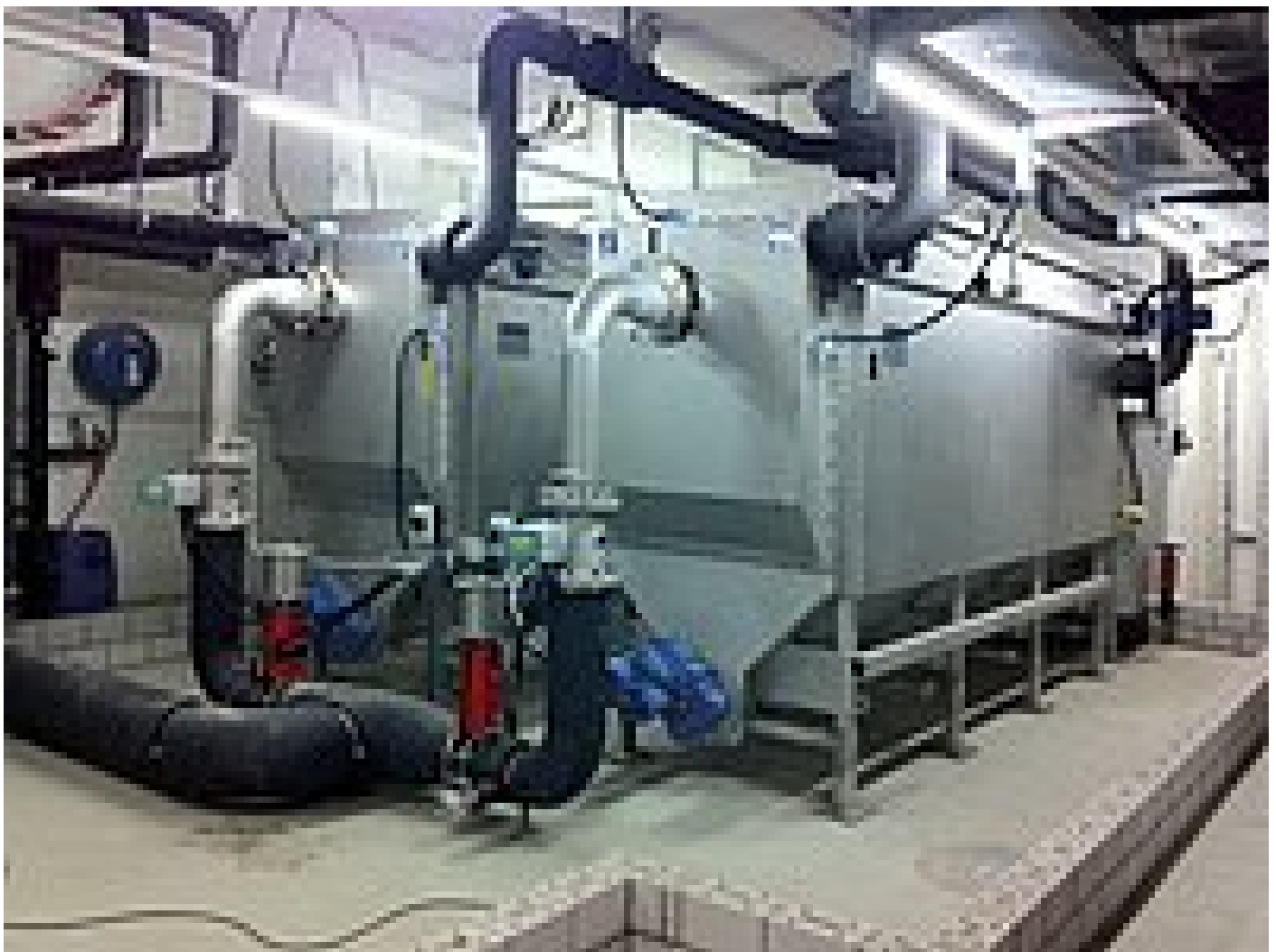
Two RoWin Heat Exchanger size 8 installed in the second basement of the Wintower building at Winterthur
