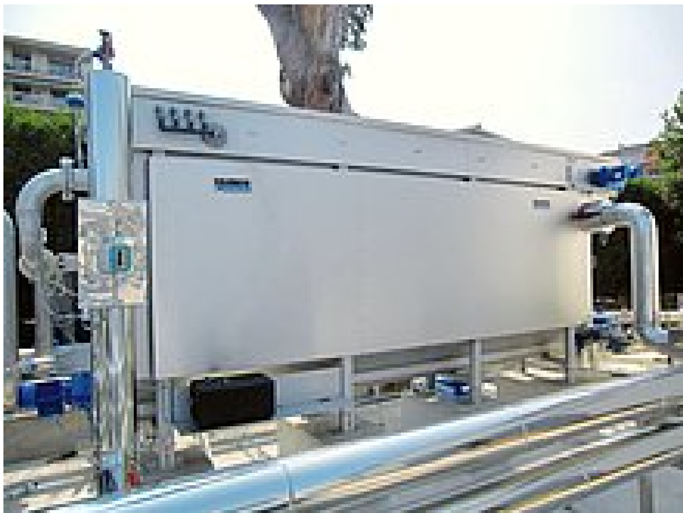
A HUBER Heat Exchanger RoWin installation on the Côte d'Azur
