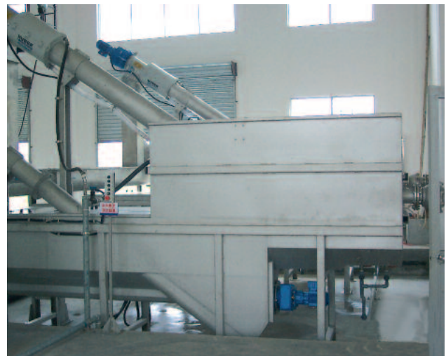
A pair of parallel ROTAMAT® Ro 3.3 units in Dong Guan, China
