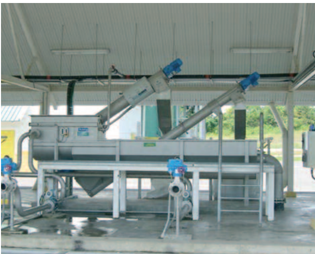
ROTAMAT® Ro 3.3 septic sludge pre-treatment unit in Kuching, Malaysia
