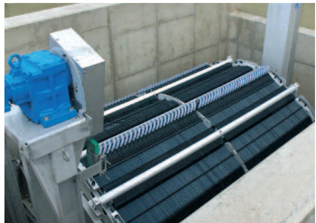
Slowly rotating HUBER VRM® ultra-filtration membrane in a membrane bio-reactor
