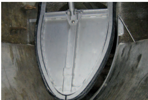
Flushing gate installed in a manhole, egg-shaped profile 1200/800
