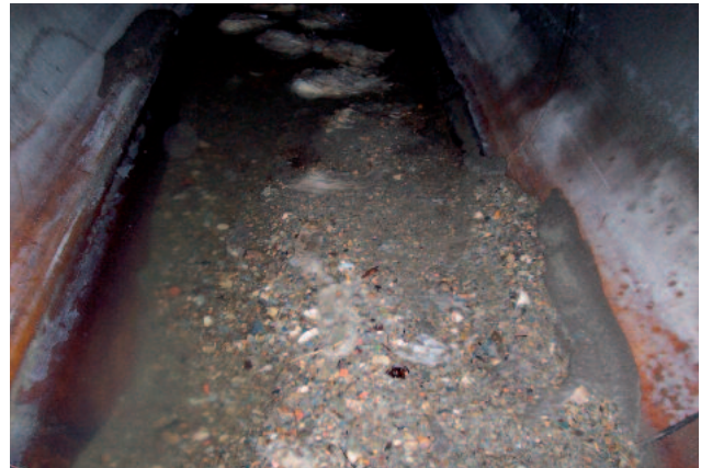
Extensive hardened sediments on the sewer bottom
