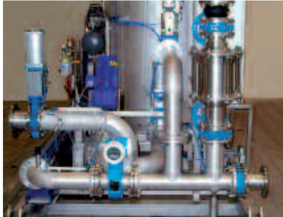
Optimised sludge digestion
