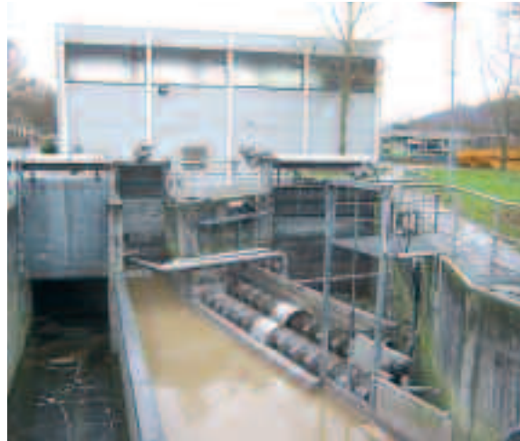
Combination of different screening systems for optimised treatment of large volumes of wastewater
